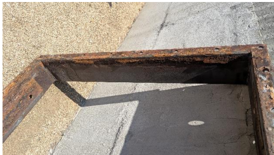
Figure 4: Corroded gate frame
