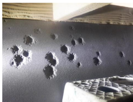
Figure 2: Deep pitting inside hopper
