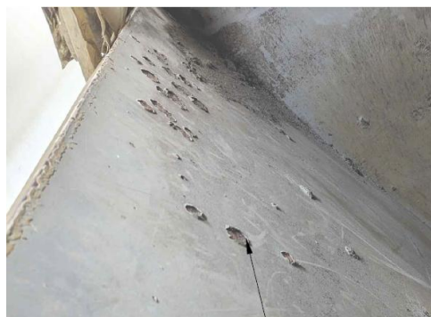
Figure 1: Corroded areas inside hopper
